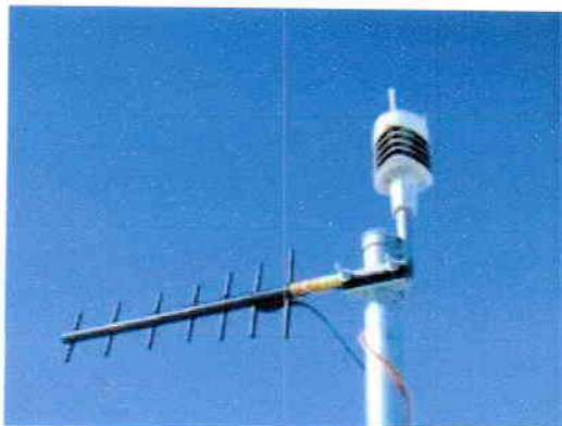
Weather sensor and cell antenna:
